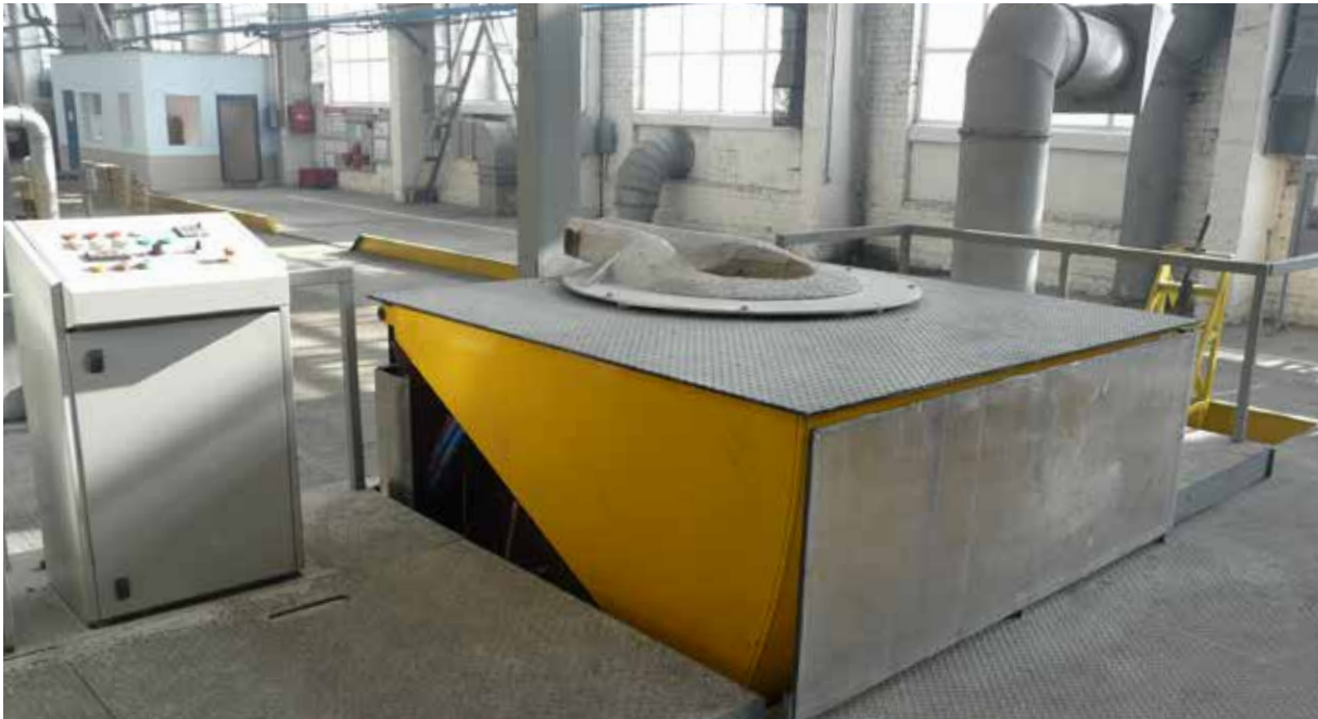
A new 1,200 kg-capacity FIB furnace being installed at a bearing manufacturer's facility.
