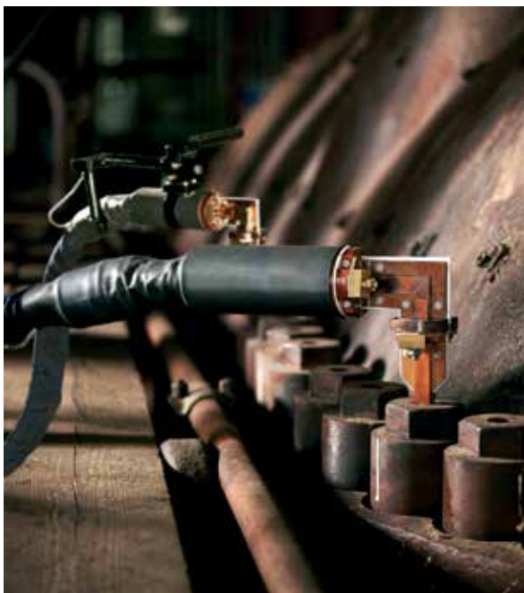
An example of shrink fitting—EFD Induction equipment removes large nuts and bolts in a fraction of the time needed by traditional gas or resistance heating.
