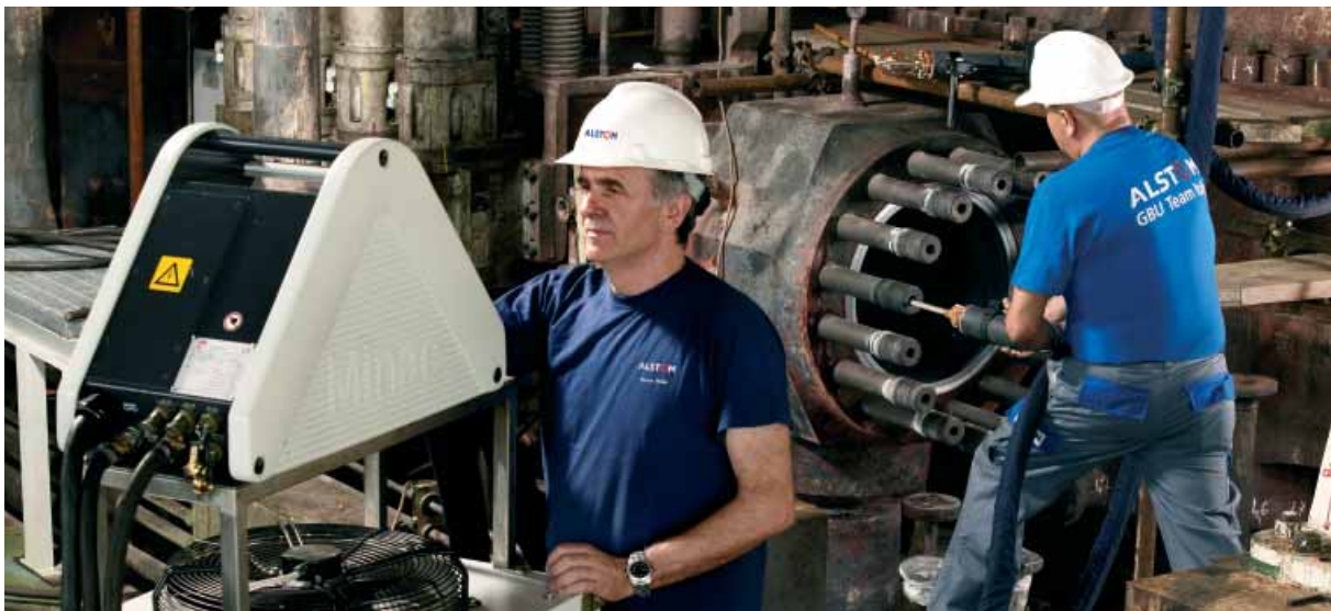
An EFD Induction Minac 25/40 Twin heating bolts on a steam turbine. This particular model features two independent handheld transformers, both powered by one compact and maneuverable converter.
