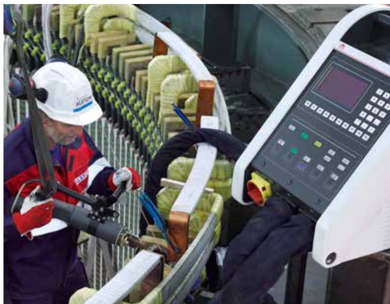
An EFD Induction Minac brazes generator windings. Minac's mobility and the handheld transformer let operators access hard-to-reach areas.
