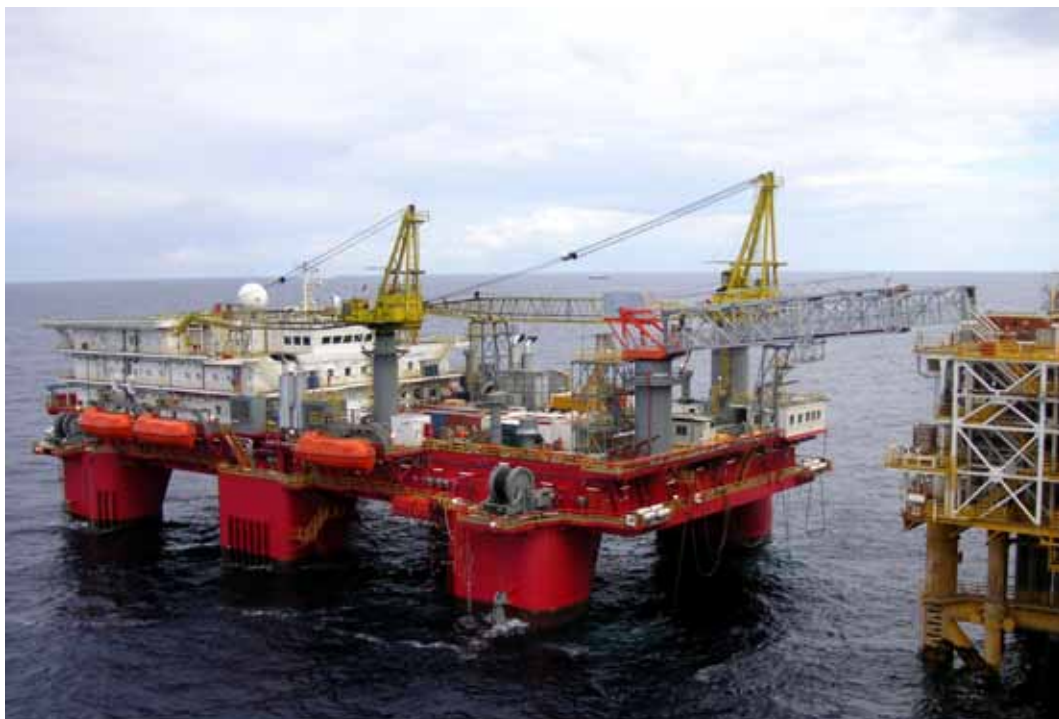
The 'Safe Concordia' accommodation and support platform. A mobile EFD Induction Minac system was used to pre-heat the weld area during the welding of a patch onto a crane tower.
